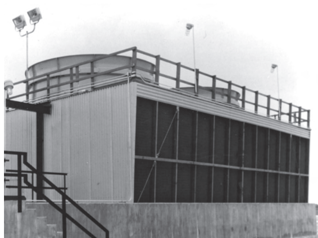
Figure 76 — Crossflow air inlet face. (Note apparent lack of louvers.)
