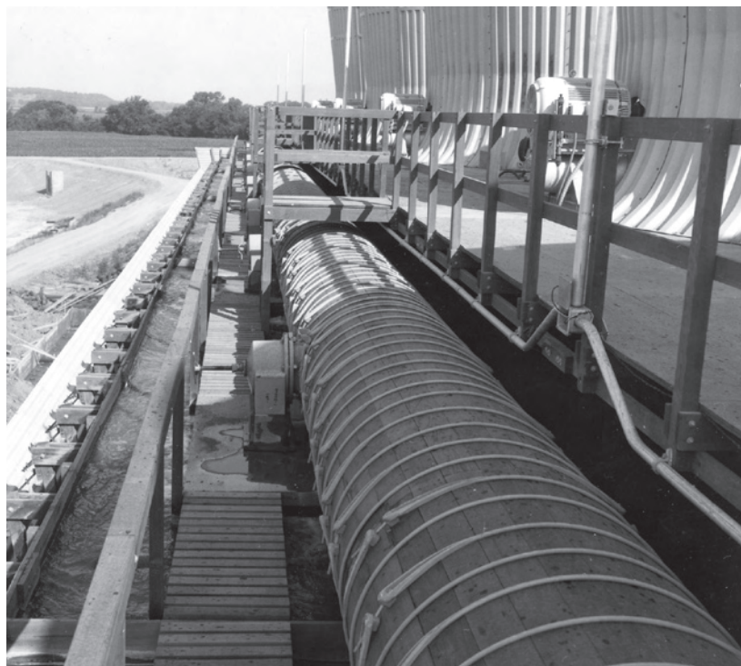
Figure 130 — Ladders, guardrails, and access-ways on a crossflow tower. Note wood stave pipe header (no longer current).
