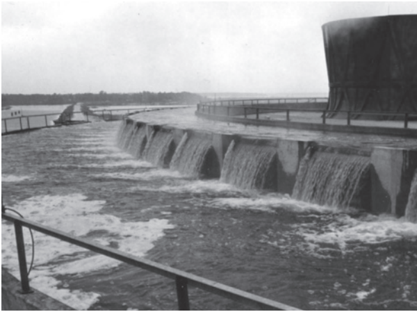
Figure 62 — Distribution system of an operating round crossflow tower.
