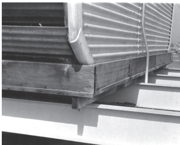
Figure 48 — Steel grillage supporting tower equipped with wood cold water collection basin.
